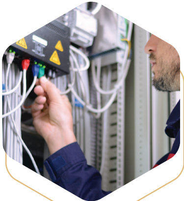
FIBER OPTIC NETWORK
